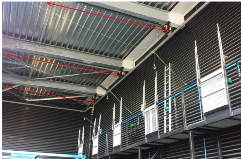
T-Lines installed under the canopy in the 3 bays where access is required.
