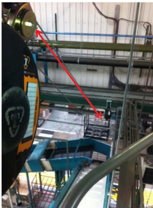
T-Line mounted above the conveyor, with each end at different heights
