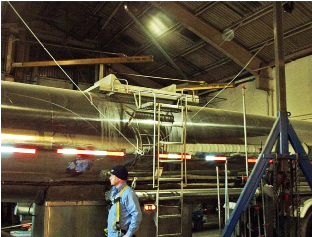
T-Line installed at Tanker Trailer Service Facility – allows the user to hook on before leaving the ground.
